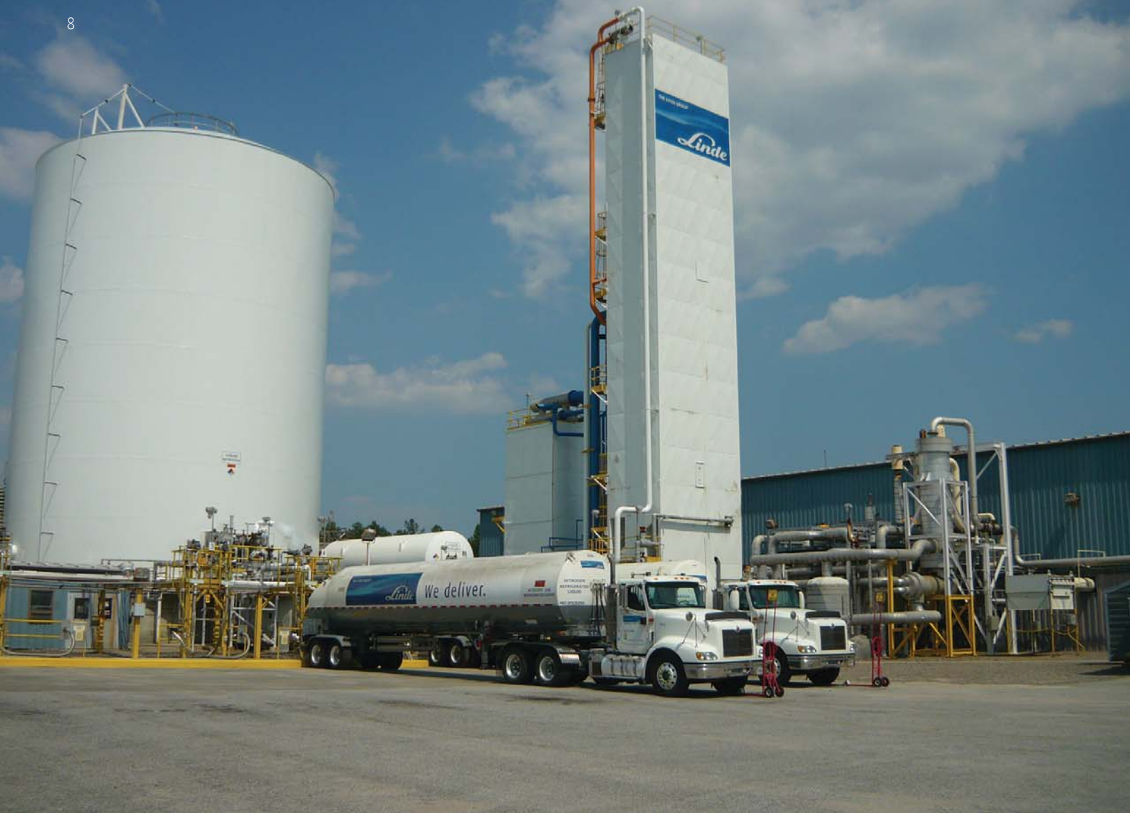
Air separation plant in Aiken, South Carolina
