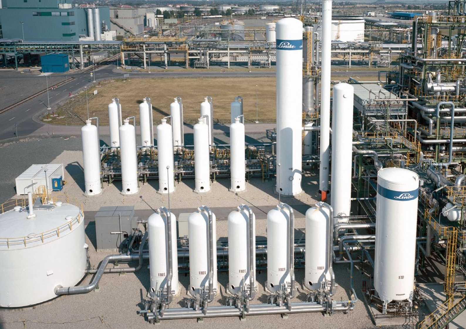
PSA units for H 2 and CO 2 recovery in a refinery in Germany
