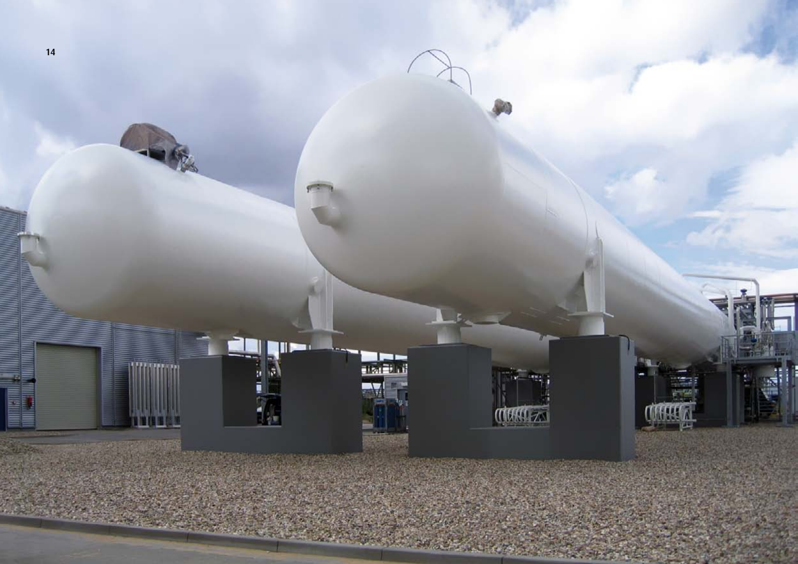
Liquid hydrogen production facility at refinery in Leuna, Germany
