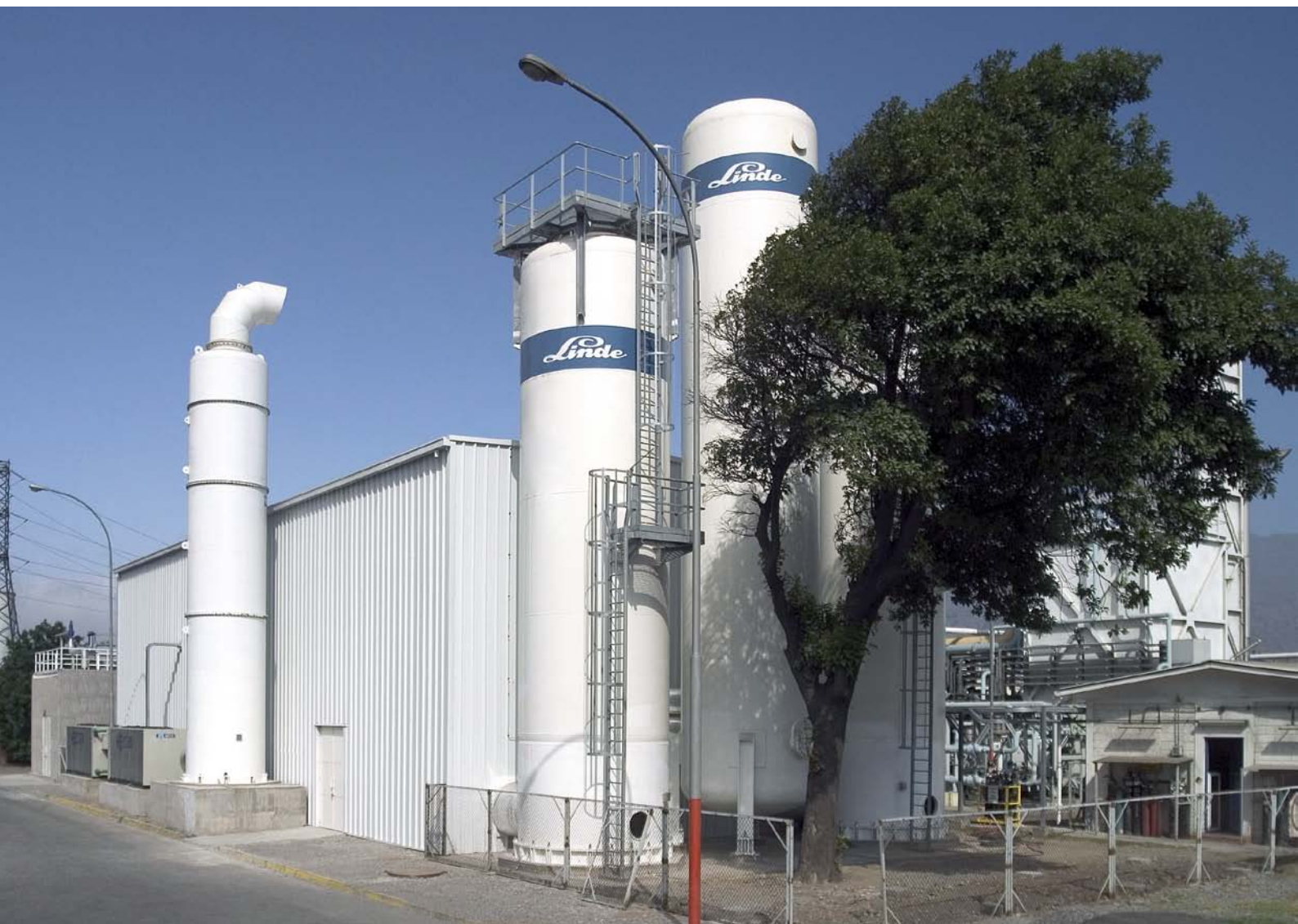
Oxygen VPSA plant in Chile
