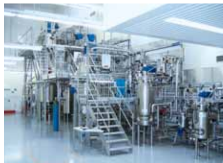
Skid-mounted modular installation
