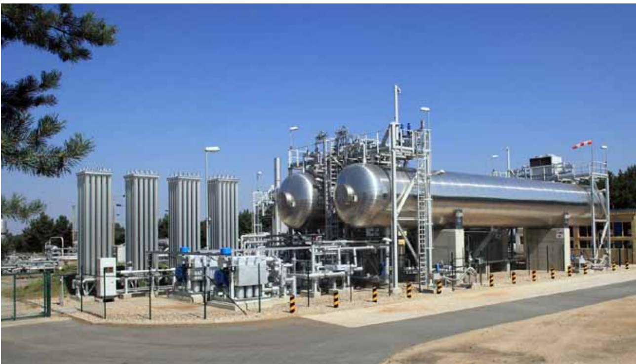
CO 2 injection plant in Maxdorf (pilot plant)
