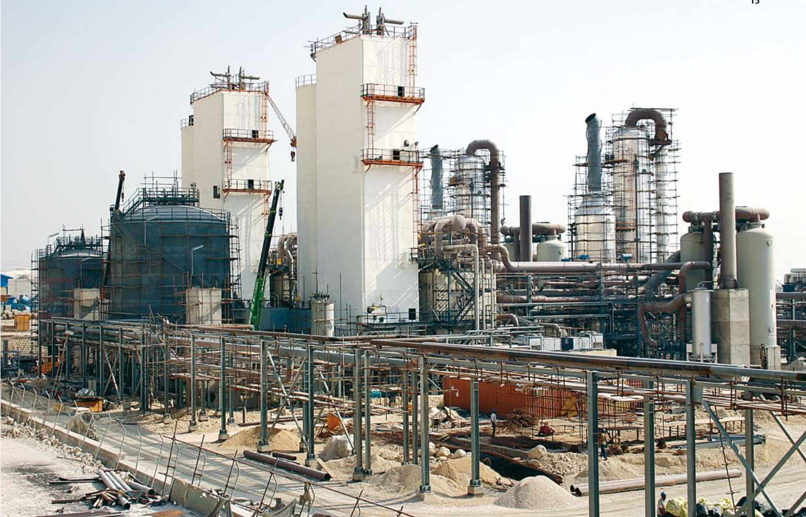
Air separation plant in Assaluyeh, Iran
