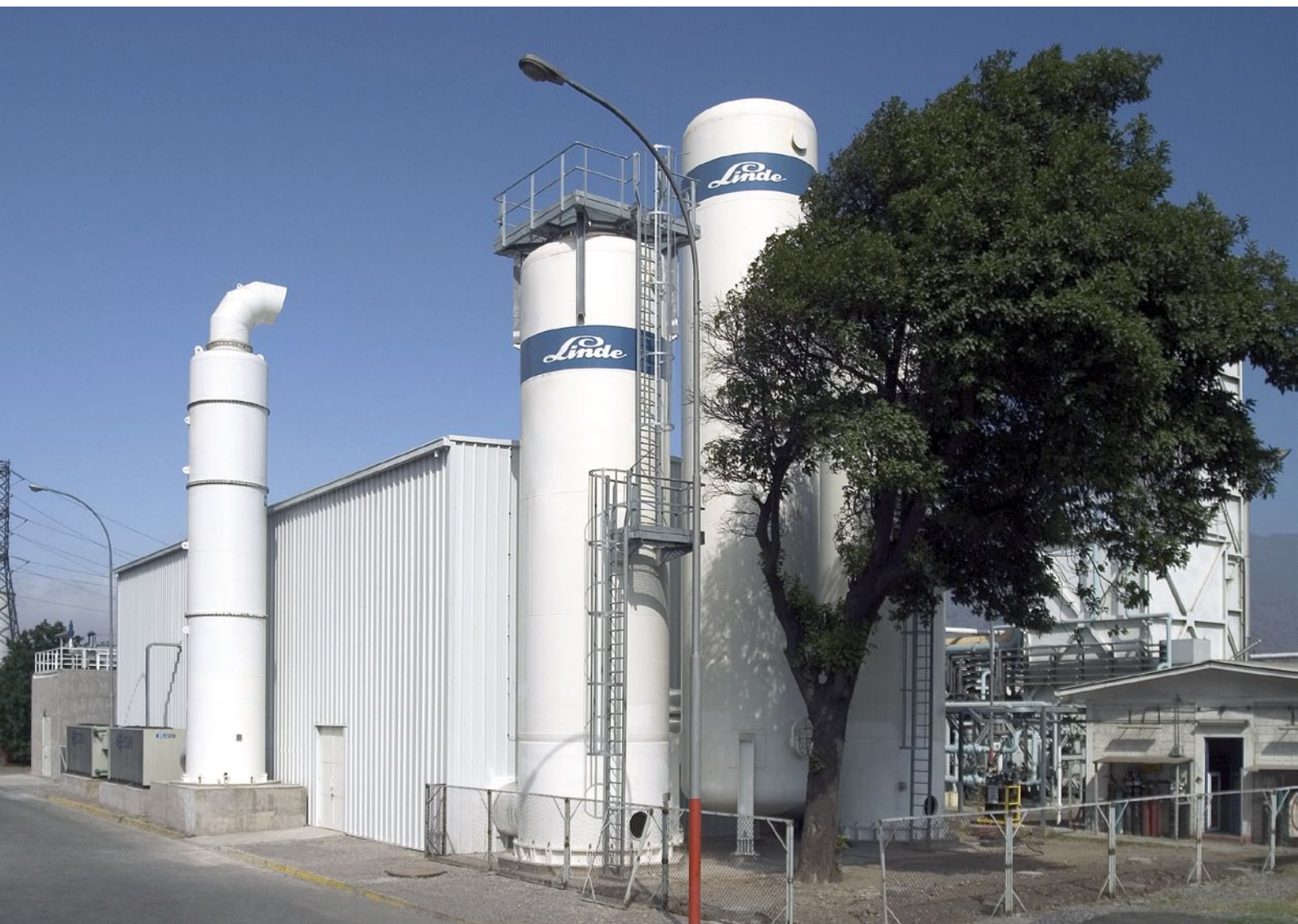
Oxygen VPSA plant in Chile
