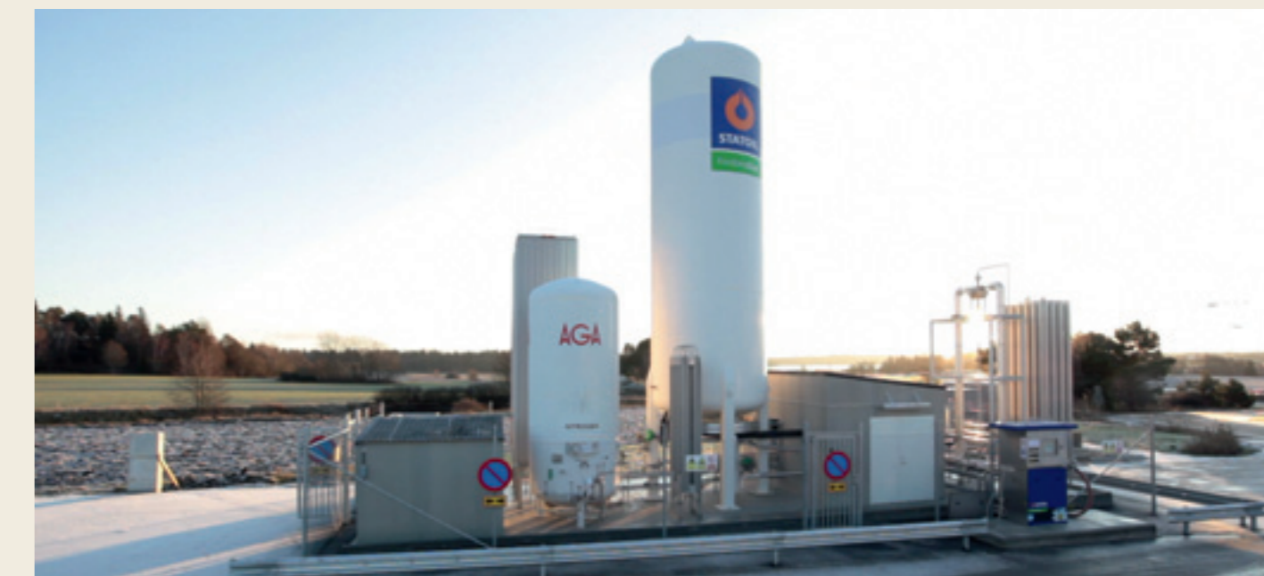
This fuelling station in Stockholm, Sweden, is equipped with a combined LNG and LCNG technology provided by Linde's subsidiary AGA.
