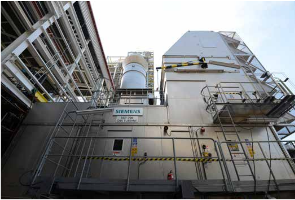
Figure 5. Siemens SGT-700 gas turbine at BOG reliquefaction plant in Bintulu.
