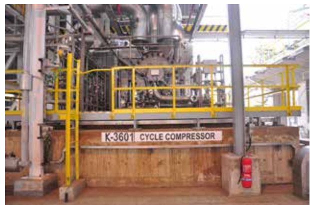
Figure 4. Siemens cycle compressor at BOG reliquefaction plant in Bintulu.
