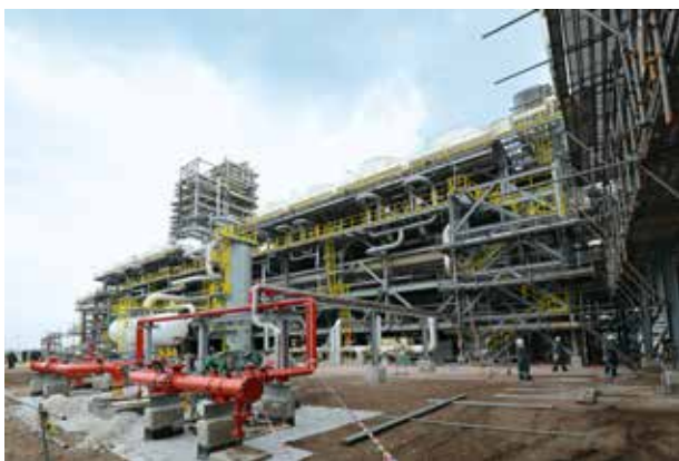
Figure 6. BOG reliquefaction plant in Bintulu.
