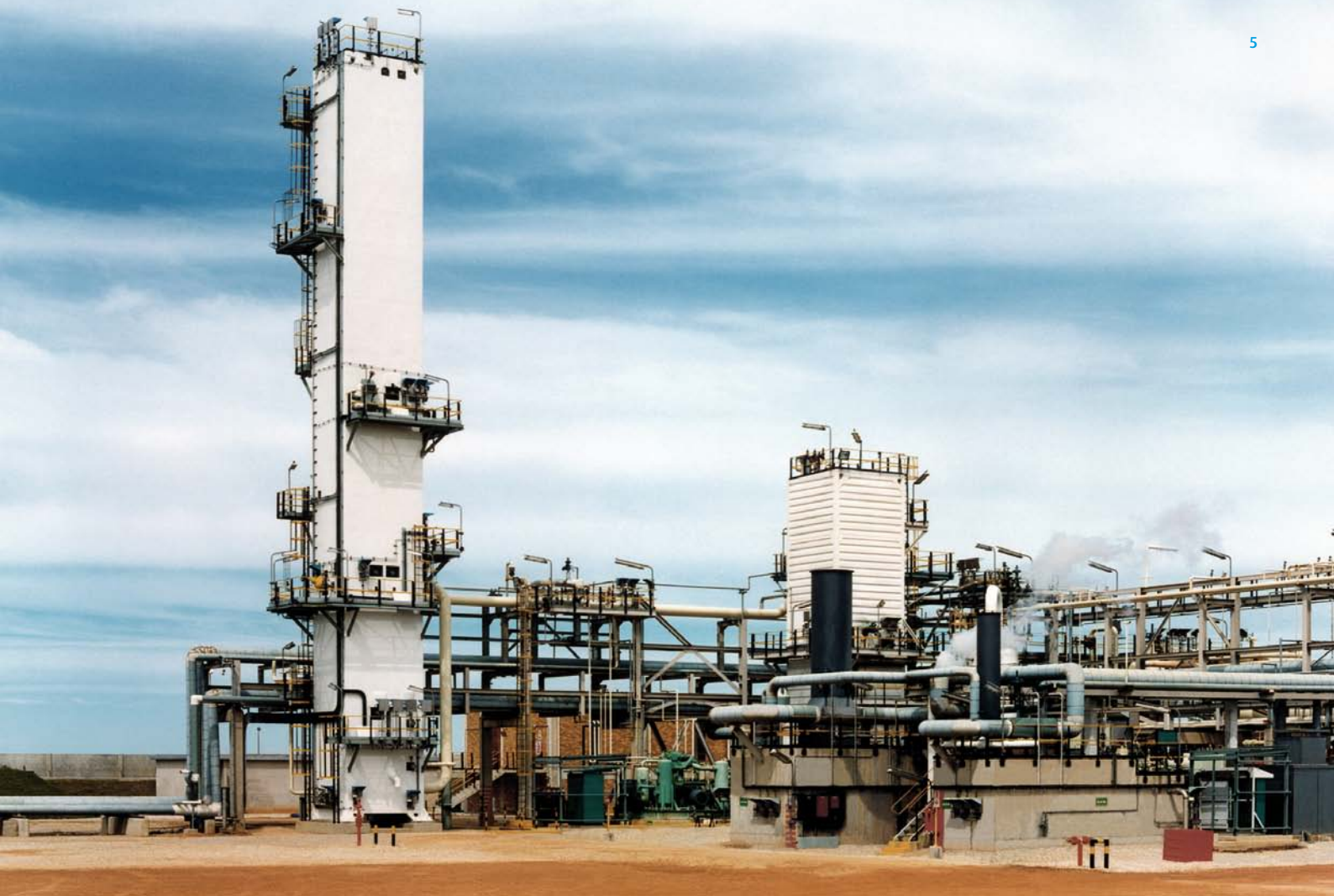
LNG (liquid natural gas) plant for Moss gas (now PetroSA) Mossel Bay, South Africa
