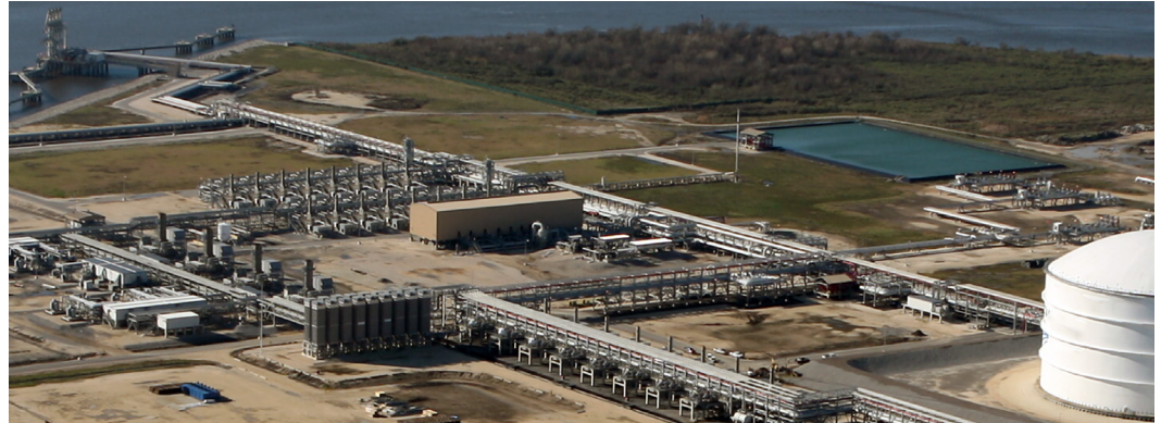
24 Sub-X ® SCVs installed at a US Gulf Coast LNG import terminal
