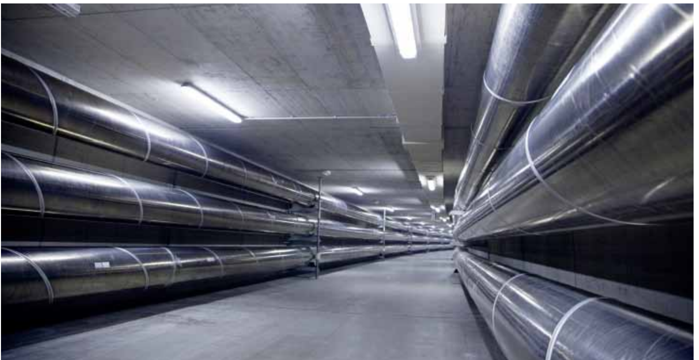
Gas-insulated high-voltage transmission line in tunnel. Reference: Siemens Erlangen, 380 KV GIL for the Paulaner brewery in Langwied, Munich.
